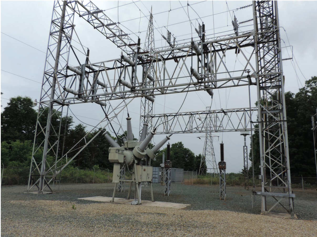
EXISTING SCOTTSVILLE SUBSTATION (VIEWING TO THE WEST)
