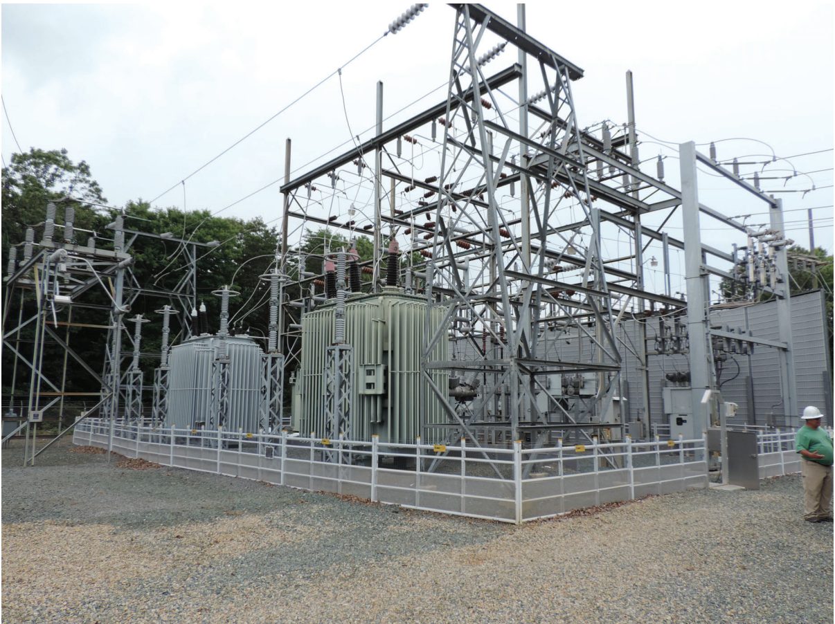
EXISTING SCOTTSVILLE SUBSTATION (VIEWING TO THE NORTHWEST)
