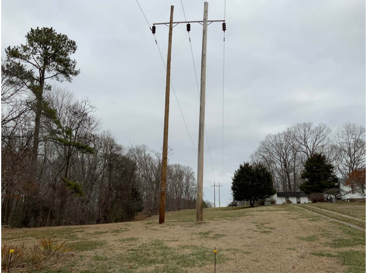
Existing H-Frame Structure Self- Supporting
